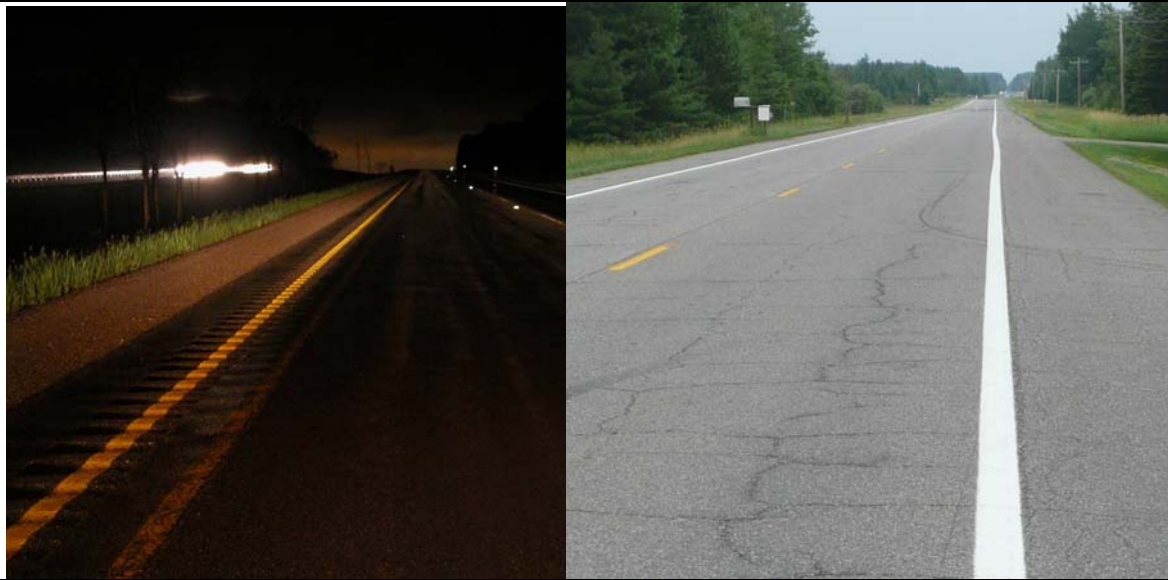
Figure 6.1 Rumble StripEs and 6 Inch Wide Edge Line
